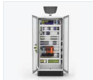
The control electronics, safety technology and industrial PC are installed in the control cabinet .
