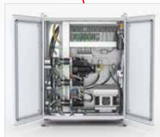
The dosing machine cabinet contains the components of the dosing periphery, e.g. the dosing pumps.
