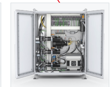
The dosing machine cabinet contains the components of the dosing periphery, e.g. the dosing pumps.
