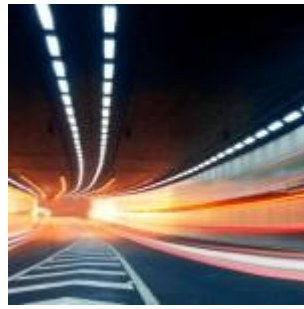
LEDs for tunnel lightings
