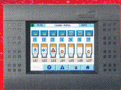
Hopper loader status
