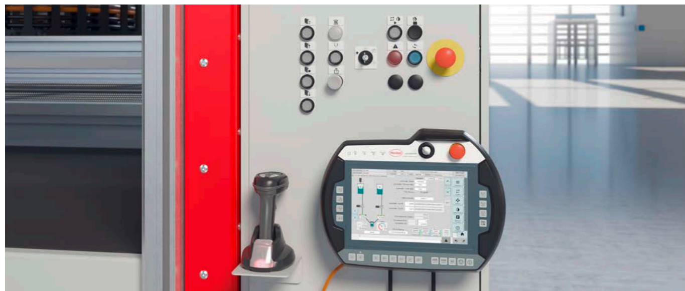
MP 2 mobile panel and above it the operating mode control panel, e.g. key switch for operating mode preselection with selection for the operating modes of Setup / Stand-by / Manual / Automatic, warning lights and EMERGENCY STOP, part of the tried-and-tested SONDERHOFF SAFETY concept.
