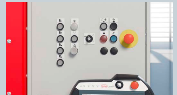
Operating mode control panel with warning lights, key switch for preselection of the operating mode, operating keys for high-speed door, and EMERGENCY STOP with proven Sondershoff SAFETY concept.
