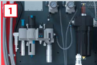
Compressed air connection, dryer and maintenance unit
